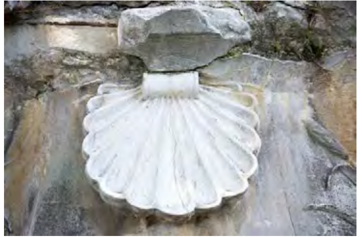
Figure 20: Shell motif condition amid limestone damage indicating restoration or replacement at some point in time
