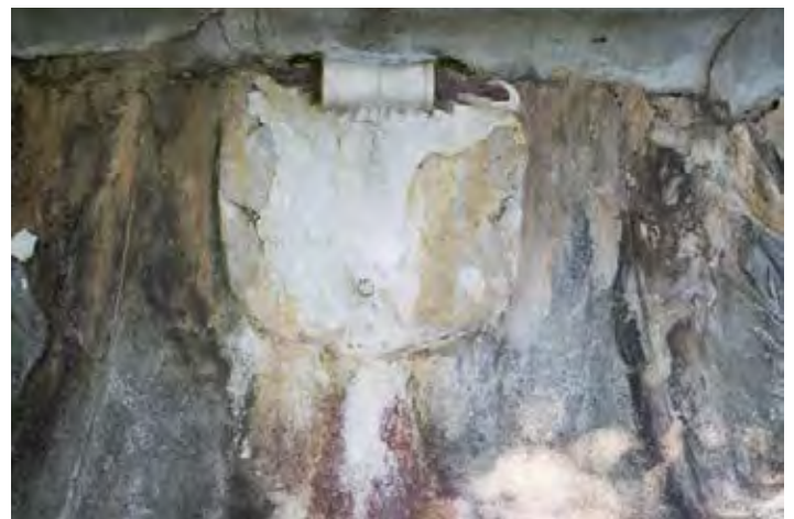
Figure 52: View of missing shell
