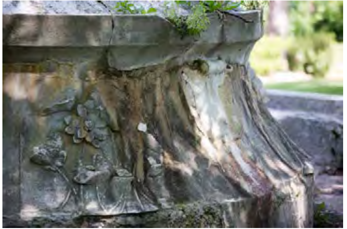
Figure 29: Excessive damage and improper repair with organic growth that is indicative of the level of disrepair
