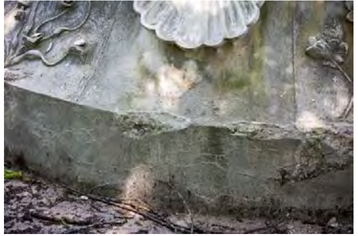
Figure 32: Degradation and mineral staining at trailing water
