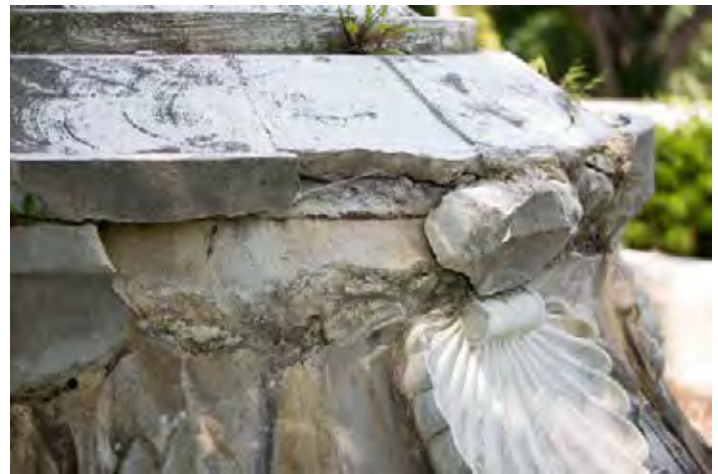
Figure 42: View of damage at tension ring
