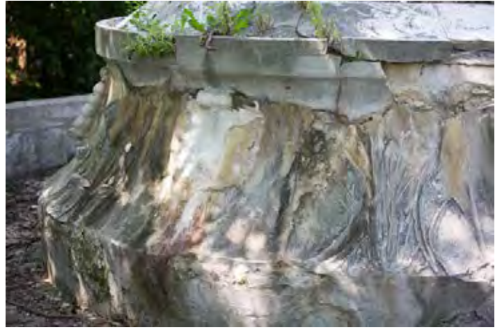
Figure 26: Excessive damage and improper repair with organic growth that is indicative of the level of disrepair
