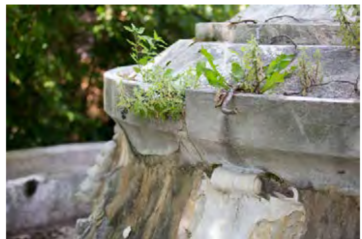
Figure 43: View of plant infestation and damage
