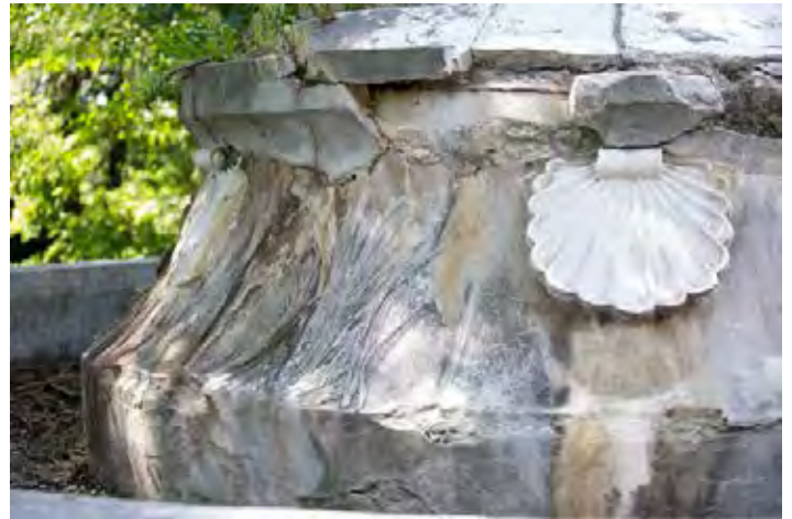
Figure 21: Excessive limestone damage adjacent to steel tension ring - causing iron oxide (rust) staining
