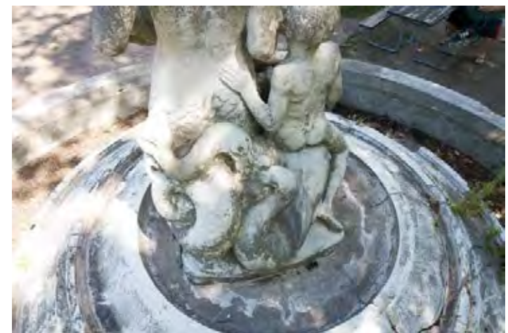
Figure 10: View of marble figures and upper view of pedestal and base - note mineral and organic buildup
