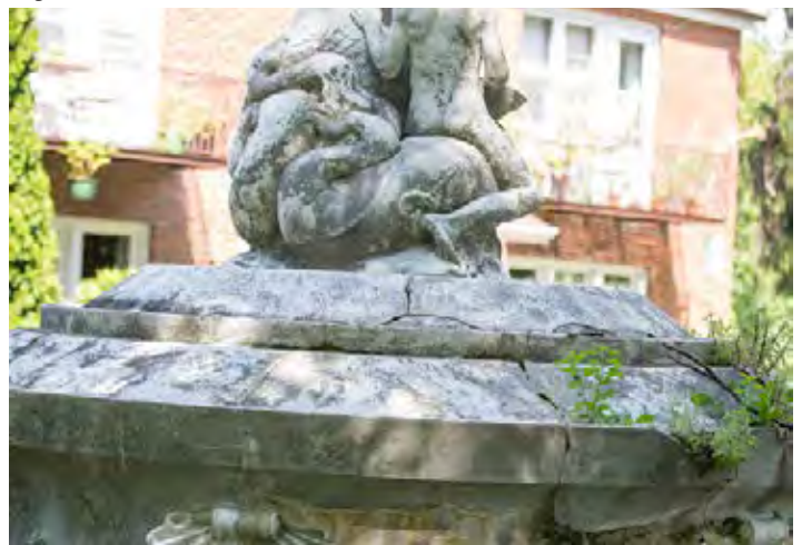
Figure 28: Close up of primary area that should be used when recreating the stone base
