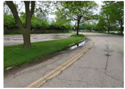
Figure 5.48. Drainage issues at South Lot
