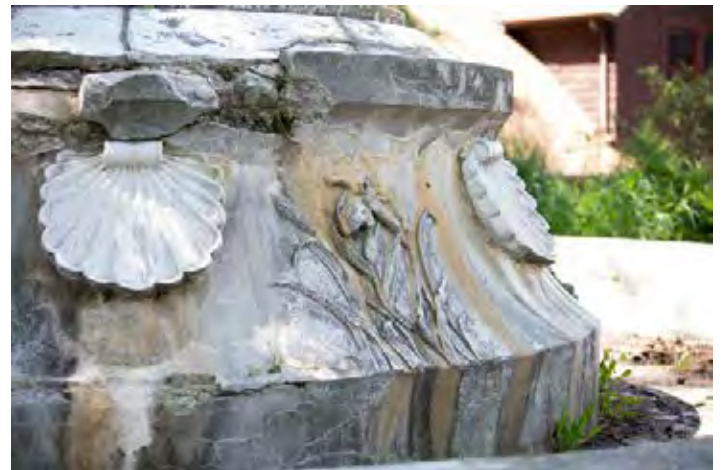
Figure 22: Overall condition of stone base - the damage is excessive and beyond repair
