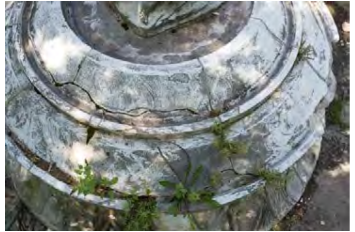
Figure 8: Upper view of pedestal and base - note damage to pedestal has been repaired and appears to have stabilized
