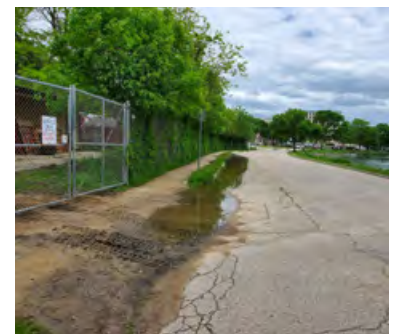
Figure 5.39. Slippage and Longitudinal
