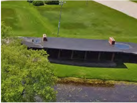
Figure 5.4. Water Ponding on Roof
