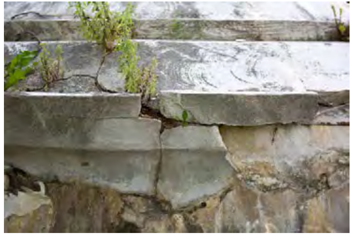
Figure 41: View of extreme damage to the limestone
