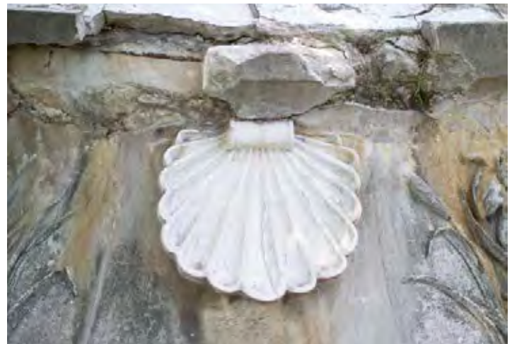
Figure 45: View of damage to limestone at base and relatively intact condition of shell motif
