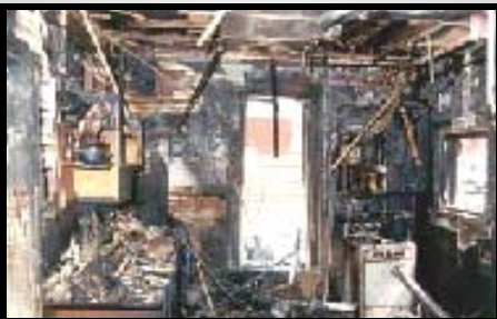
Devastation caused by a Kitchen Fire
