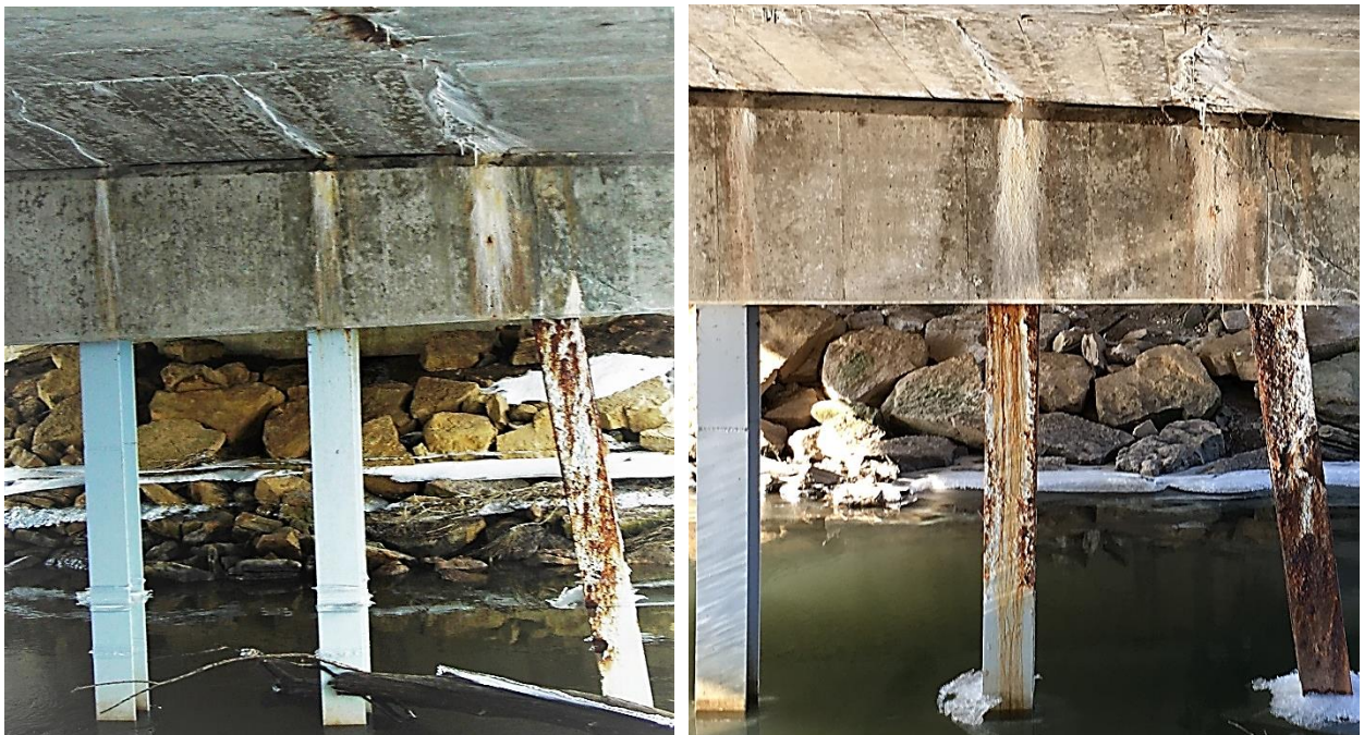
Corrosion of former Highway 19 Yahara River Bridge. March of 2013 on left, December of 2019 on right. Stalactites form at the largest fracture every winter and slowly dissolve over the remainder of the year.
