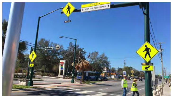
A rapid flashing beacon at a difficult crossing increases visibility of pedestrians.
