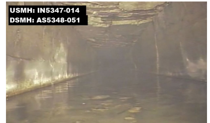
ROOF SPALLING IN AREAS BELOW TREES, EXPOSING STEEL REBAR
