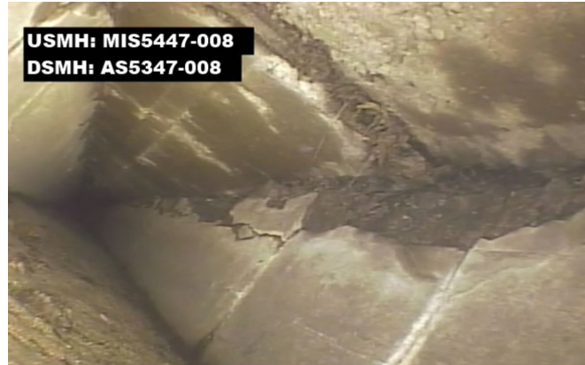
FRACTURING FROM ROOT INTRUSION
