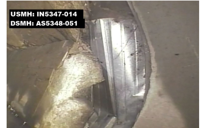
IMPROVISED PATCH REPAIRS
