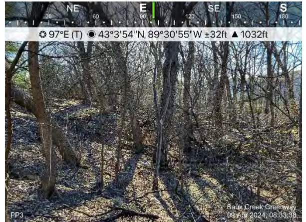
Photo #4 Photo point 3, view east in Area 1 with multiple eroded channels along wooded slope
