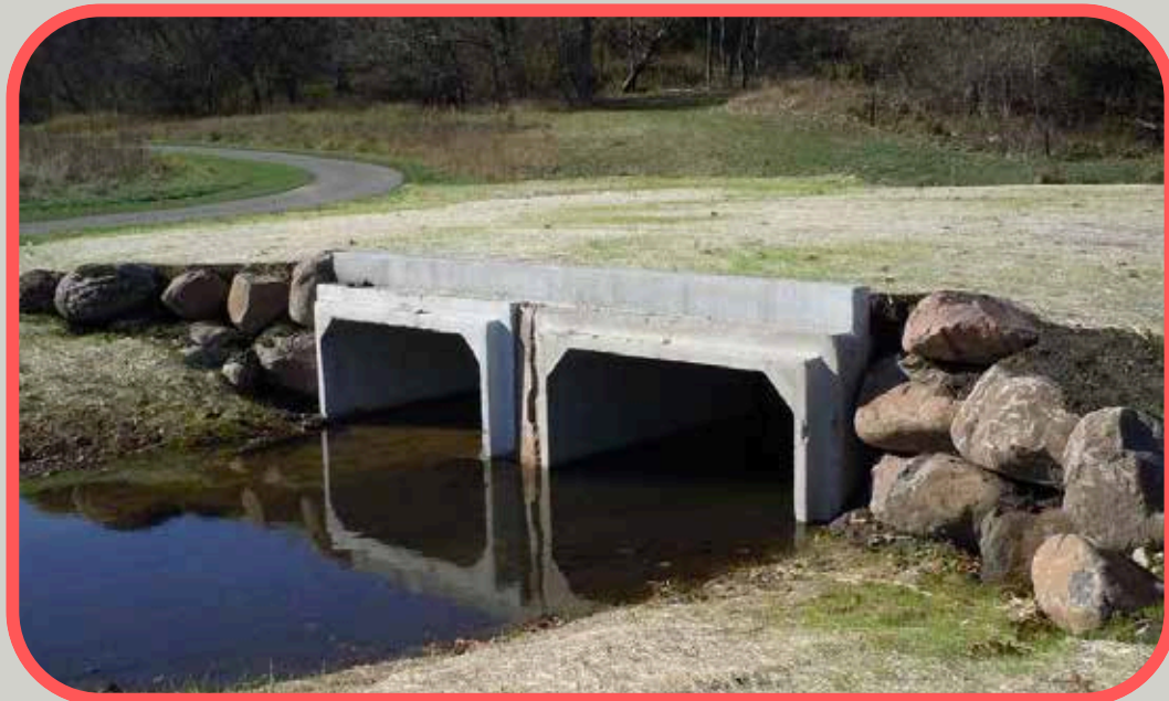
3a - Culverts at sanitary access path crossing - allows consistent and safer vector access
