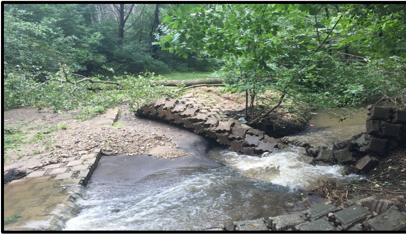
Figure 19 Failed sanitary access path
