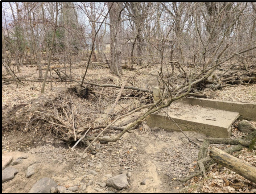
Figure 6 Concrete weir installed when pond was built to hold back water and route it into pond. The length of the concrete weir shows original width of the channel and how much it has widened.
