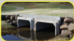
3a -Culverts at sanitary access path crossing - to allow consistent vector access. Culvert will be topped with concrete for stability
