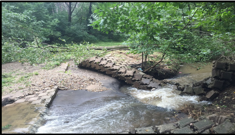
Figure 19 Failed sanitary access path
