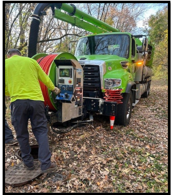
Figure 21 Vactor and crew cleaning sanitary mains via access structure in Sauk Creek greenway
