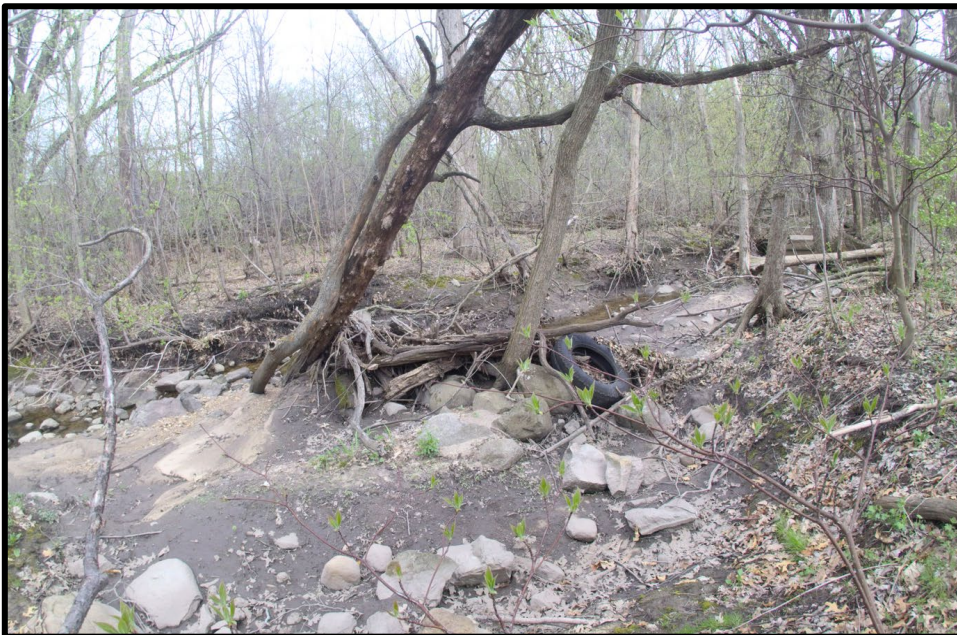
Figure 7 Channel widened due to erosion. Can see widened channel section in foreground near tire.
