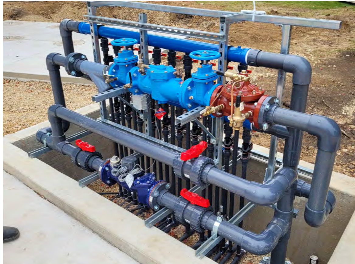
EXAMPLE SUPPLY SIDE OF COMMAND CENTER
