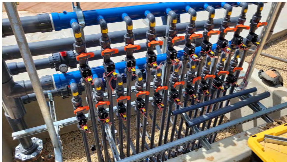
EXAMPLE MANIFOLD SIDE OF COMMAND CENTER (BY MANUFACTURER)
