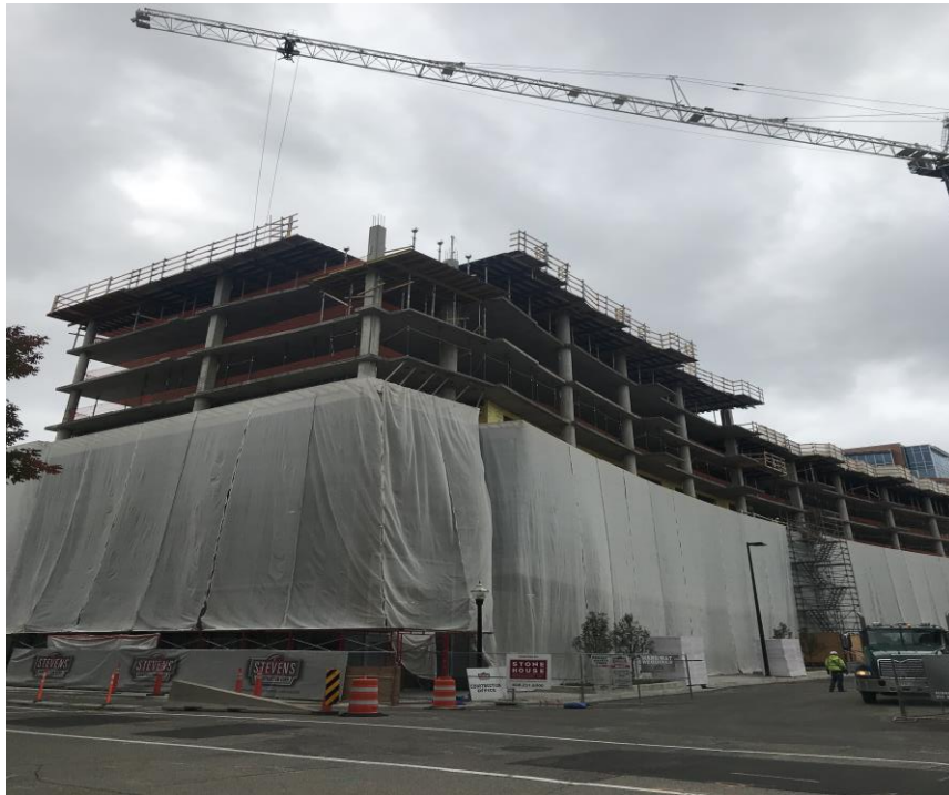
Stone House apartment construction progress on Block 88 looking north from East Wilson & Pinckney
