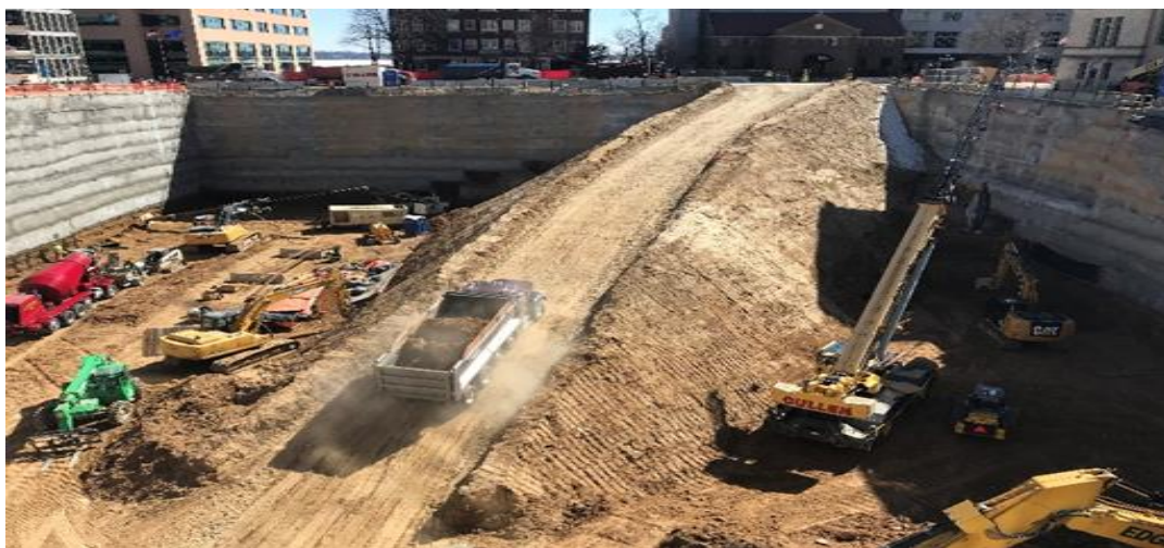
Ramp to base of the excavation. Looking South towards East Wilson Street.
