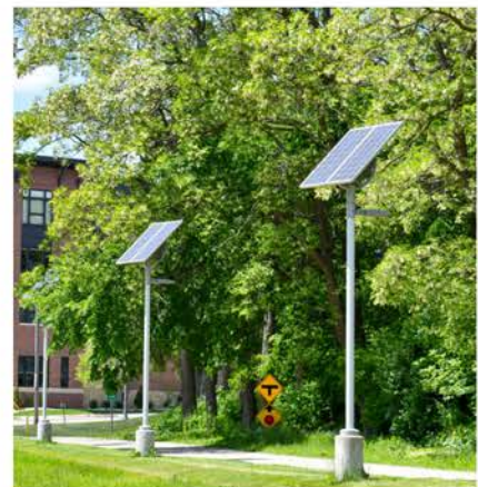
Solar lighting along the Campus Drive bicycle path
