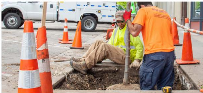
Members of the Forestry Section of the Streets Division planting a tree on South Pinckney Street
