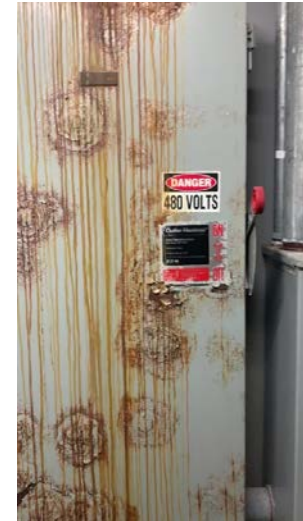
Water Damage to Main Disconnect in Room 307B (switch to be replaced by DOA project 21K2D)
