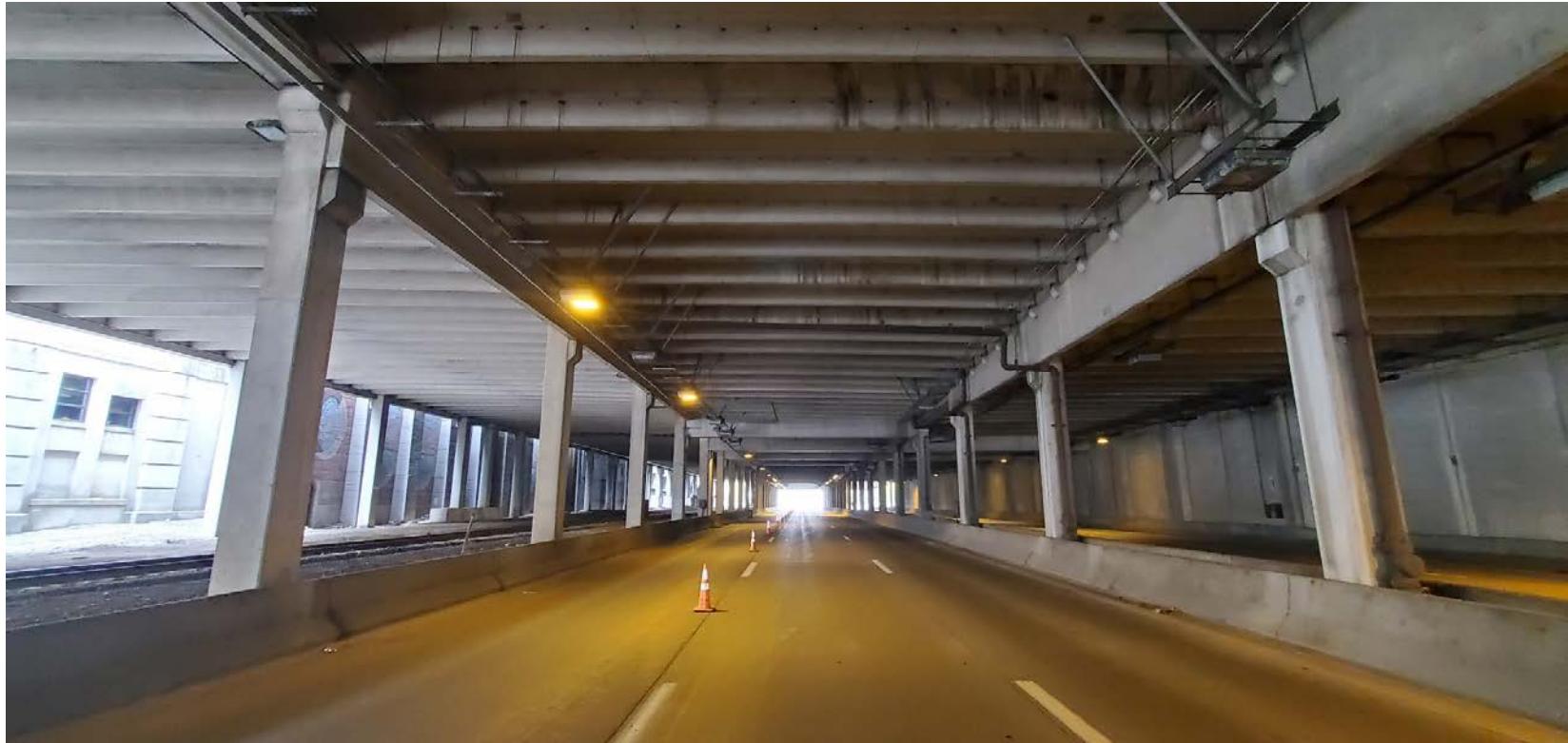
Existing Tunnel Lighting Configuration
