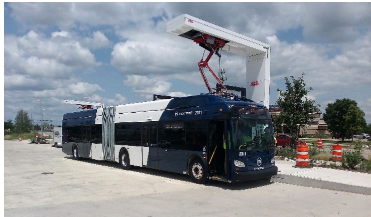
Figure 32 New Bus Charger for Batterie Electric Buses
